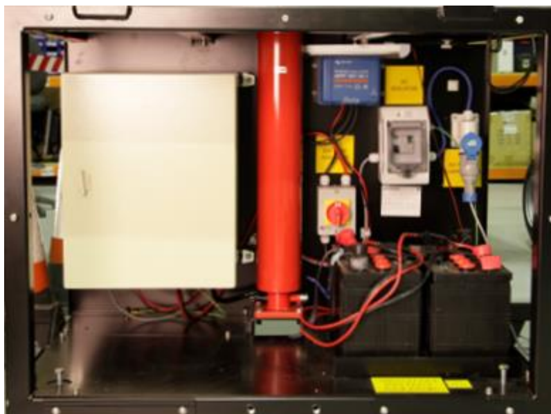
Figure 5 - Inside the Main Enclosure
